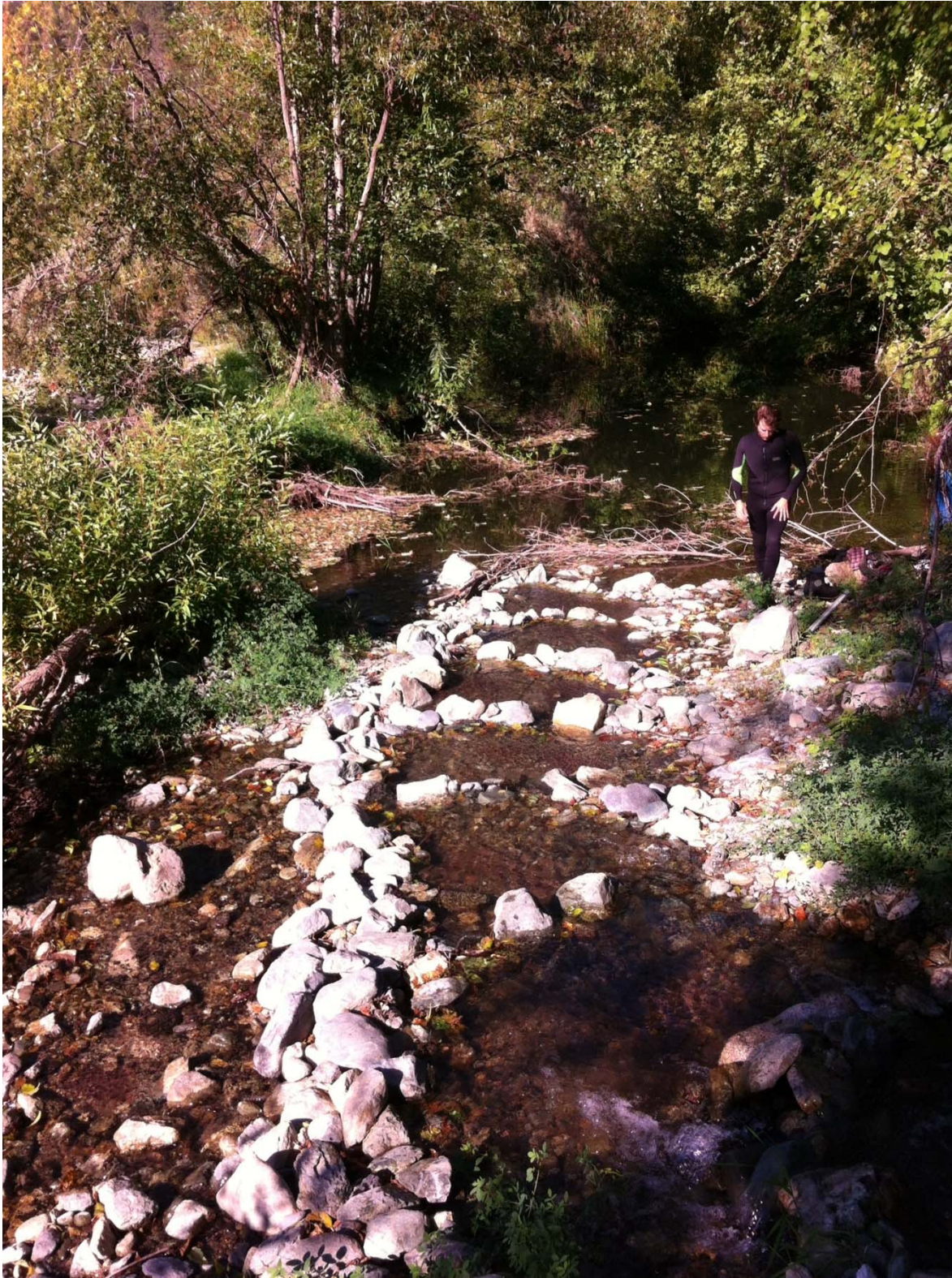
Photo 3. Downstream view of second berm-lined channel directing portion of Stanshaw Creek flow to the floodplain pond. The pond outflow, obscured by bushes, is to the left. Note the flow going under the rock berm to the left. That flow passes directly to the Klamath River
