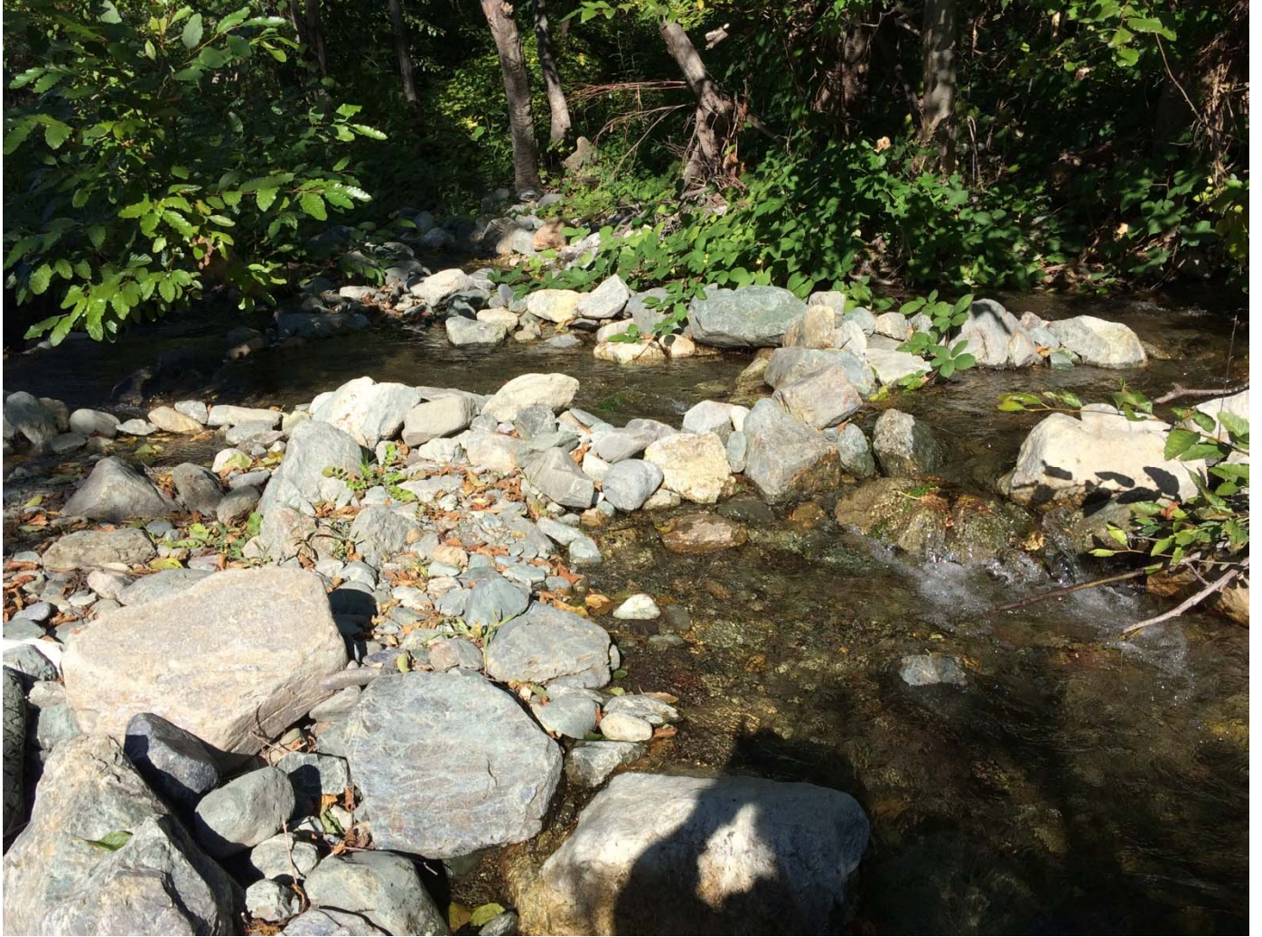
Photo 1. View looking upstream at the location where Stanshaw Creek emerges from its confined channel and enters the active floodplain of the Klamath River. The velocity energy of the channel is toward the right in this picture, but rocks were hand-placed at the head of that channel to block its flow, and a continuing berm of rocks was placed along flow directed toward the left in this picture. The floodplain pond is about 45 feet to the left and 5 to 8 feet downslope from this picture. The next photo shows the view down one of two channels directed to the pond.
